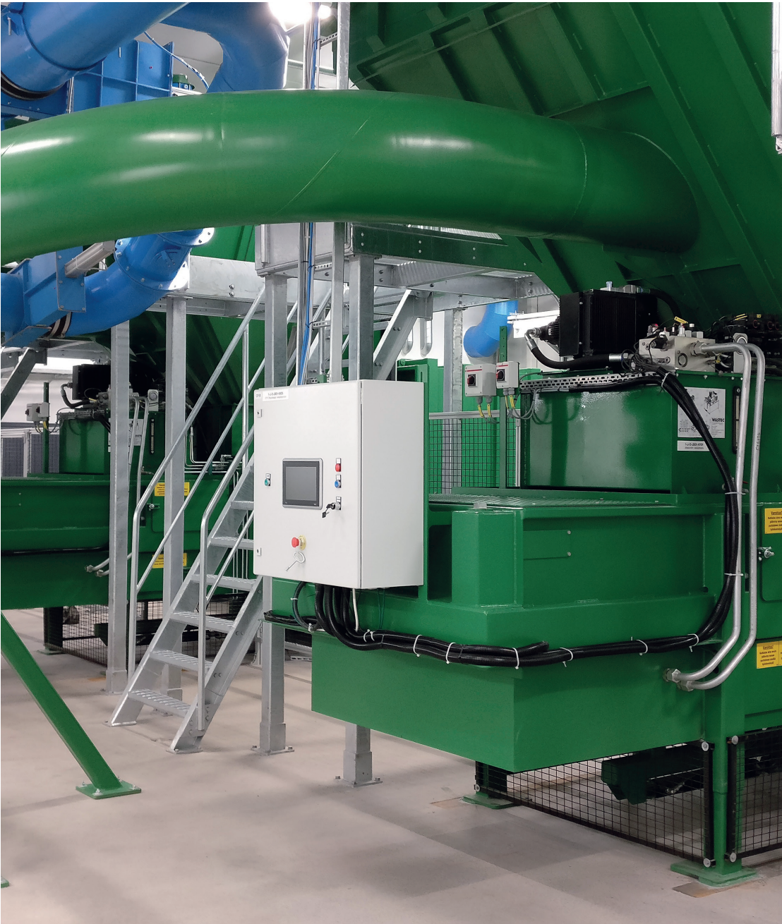
Pipe network inside an Envac terminal
