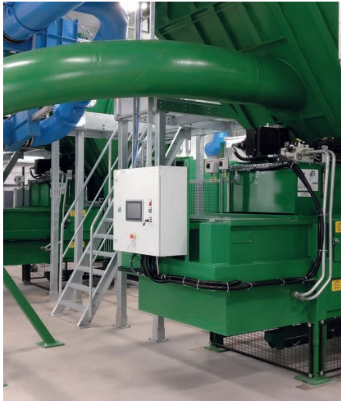
Pipe network inside an Envac terminal
